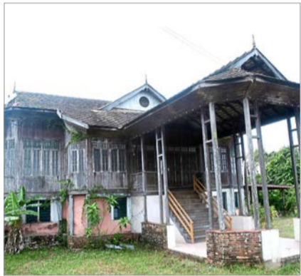
A 100-year-old traditional Malay house near Kampung Losong Haji Su at Kuala Terengganu.
