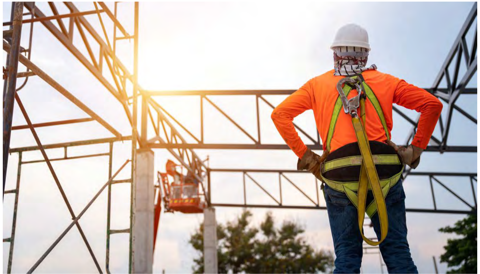
A construction worker with safety equipment to prevent falling from height at construction site.
